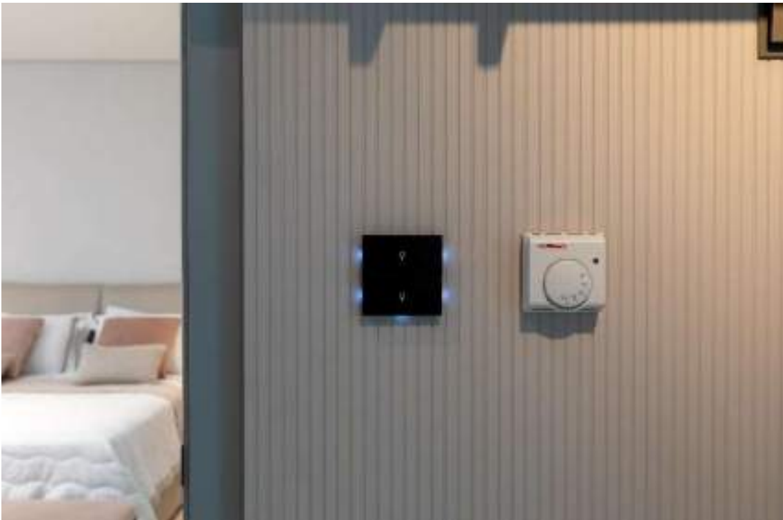
Floor Heating Thermostat
