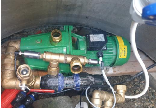
The pump for garden watering (irrigation)
