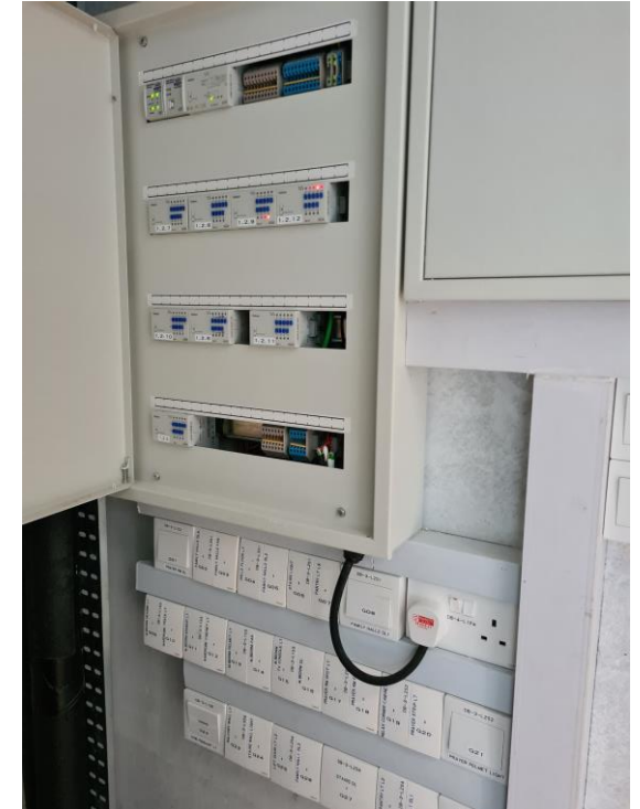
KNX Panel @ Upper Floor
